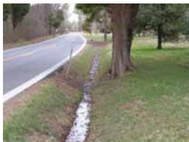
Photo 119 - Royal Oak Road, Northwest (Note Blocked Culvert Downstream)
